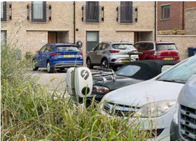
Provision of EV charging points at key places to facilitate more sustainable transport mode (Wolvercote Mill, Oxford).
